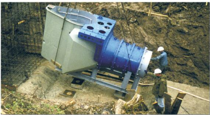
Instalace turbíny VC 1220 do MVE Kulišėnai (Litva) Installation of turbine VC 1220 into small hydro power plant Kulišėnai (Lithuania) Монтаж турбины VC 1220 - МГЭС Кульшенай (Литва)
