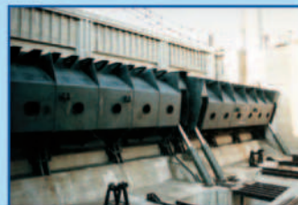
• Supported weir gate
